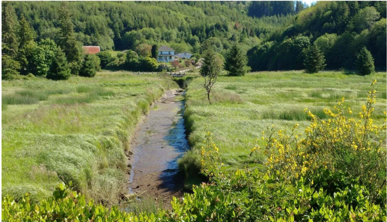
Image 5: A large ditch splits the project site into the phase 1 and phase 2 sections (see attached project map). There is a failed, collapsed culvert at the far end of this ditch to be removed in the project. Sections of the main ditch will also be filled, and a new breach will be created to reduce flow through the RR ditch and increase tidal channels in this portion of the project area. (Photo: Laura Brophy)
